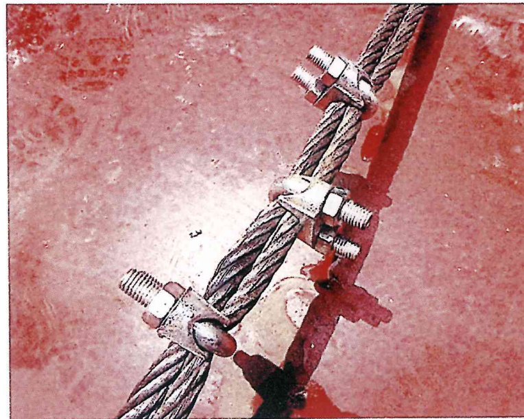
✘ Incorrect use of bulldog grips
