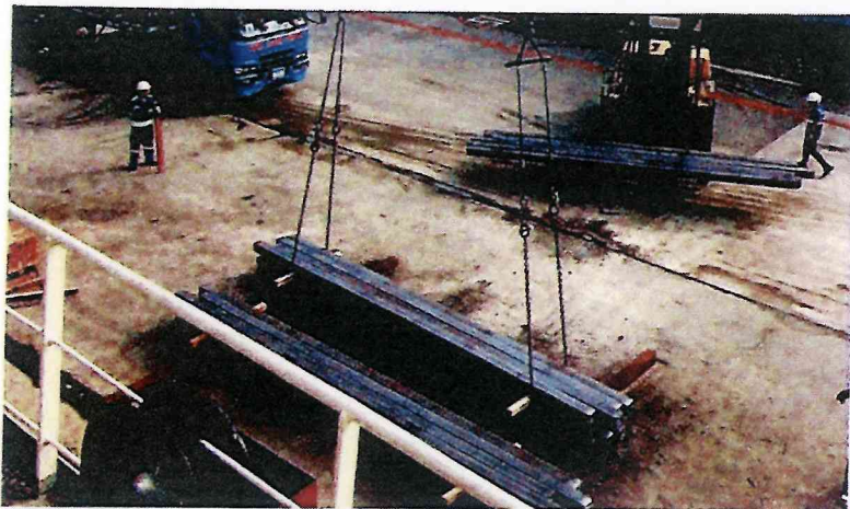
✓ Discharging blooms with the use of a single chain-leg basket lift under a spreader
