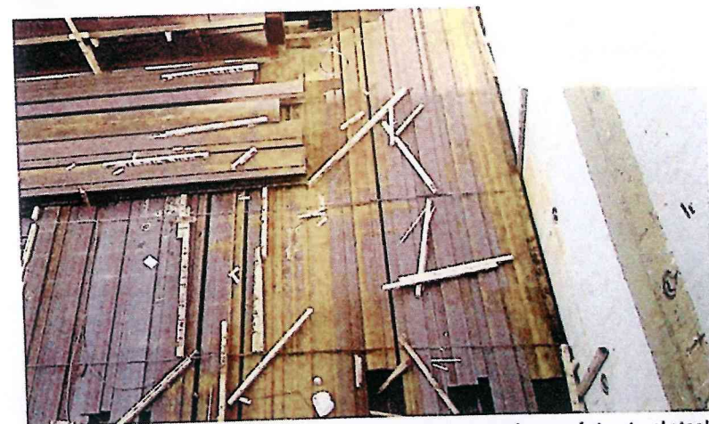
✗ 60 mm x 60 mm plywood dunnage being laid between layers of structural steel. The dunnage should be of hardwood for the first six tiers
