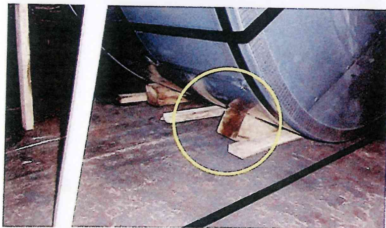
✘ First tier of coils. Incorrect place for the wooden wedge on the tank-top, but correct positioning with the right angle up
