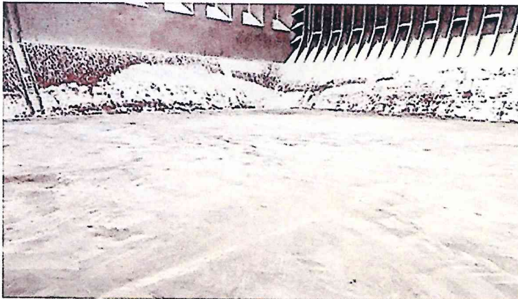
✗ Poorly prepared cargo hold on a bulk carrier. Residue from some bulk cargoes can react with, and damage, steel cargo. A silver nitrate test should be carried out to identify the presence of chlorides
