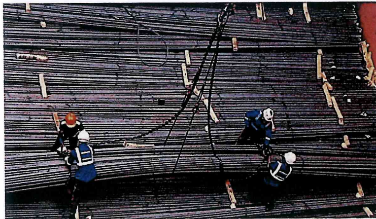
✓ Lifting the middle part of the rebar bundle, with the use of a wire, to pass the choke hitch sling. The dunnage assists in passing the lifting wire underneath
