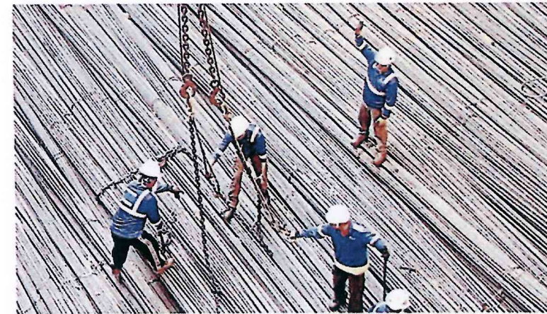
✓ Once the lifting chains are in place, the short wires are removed
