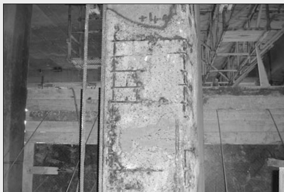
Degradation shown on a pillar due to the marine environment (© Christine RAYNAUD - BTM)
