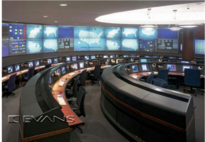
Fig. 13.3 Example of a Network Operations Center (NOC) (Reproduced with permission from Evans Consoles Corporation)
