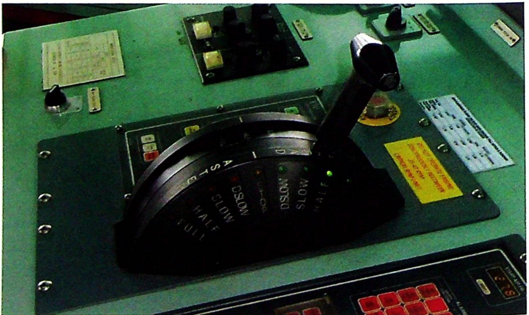
A typical telegraph and main engine control panel
