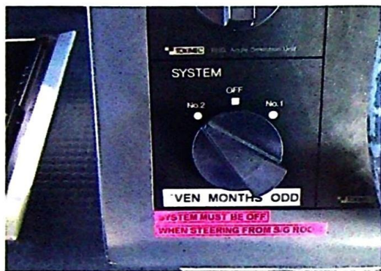
The steering system selector switch
