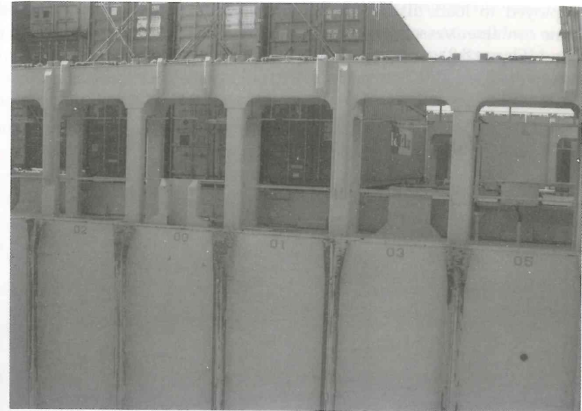
Fig. 8.1 Empty cell guides numbered odd to starboard and even to port, situated at the fore end of the cargo container hold.
