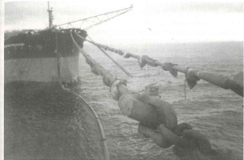
Fig. 5.15 Moorings and floating oil-bearing pipeline seen extending from the FSU 'Zapro Producer'.
